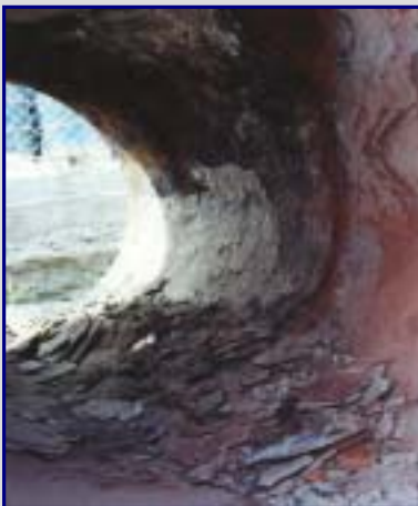
Corrosion in a duct
