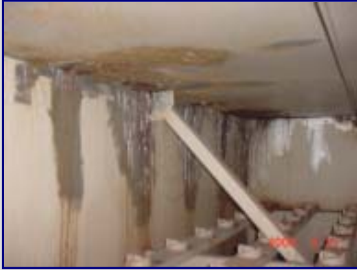
Corrosion in baghouse
