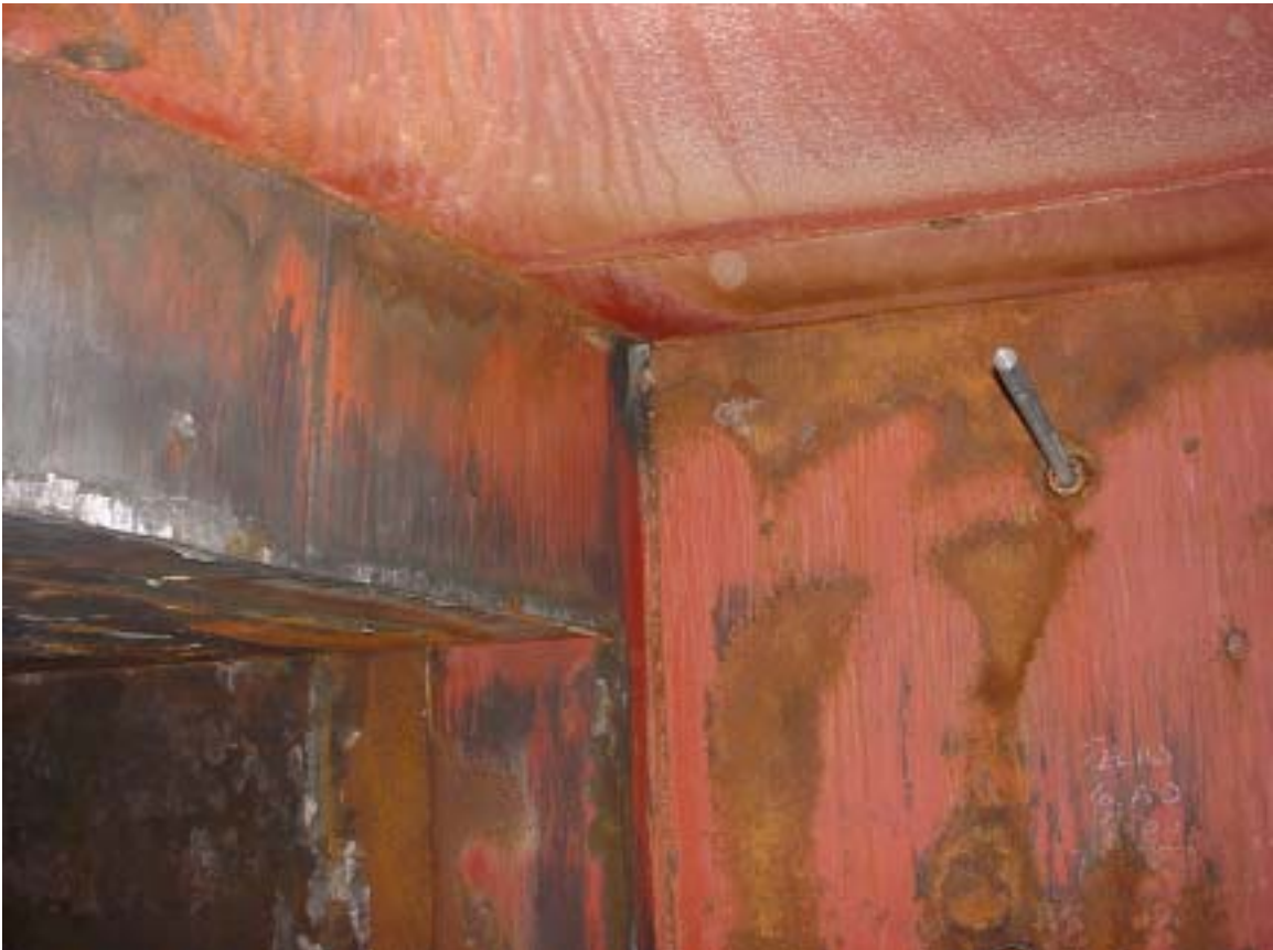
Figure 3. Corrosion damage after only six months of service.
