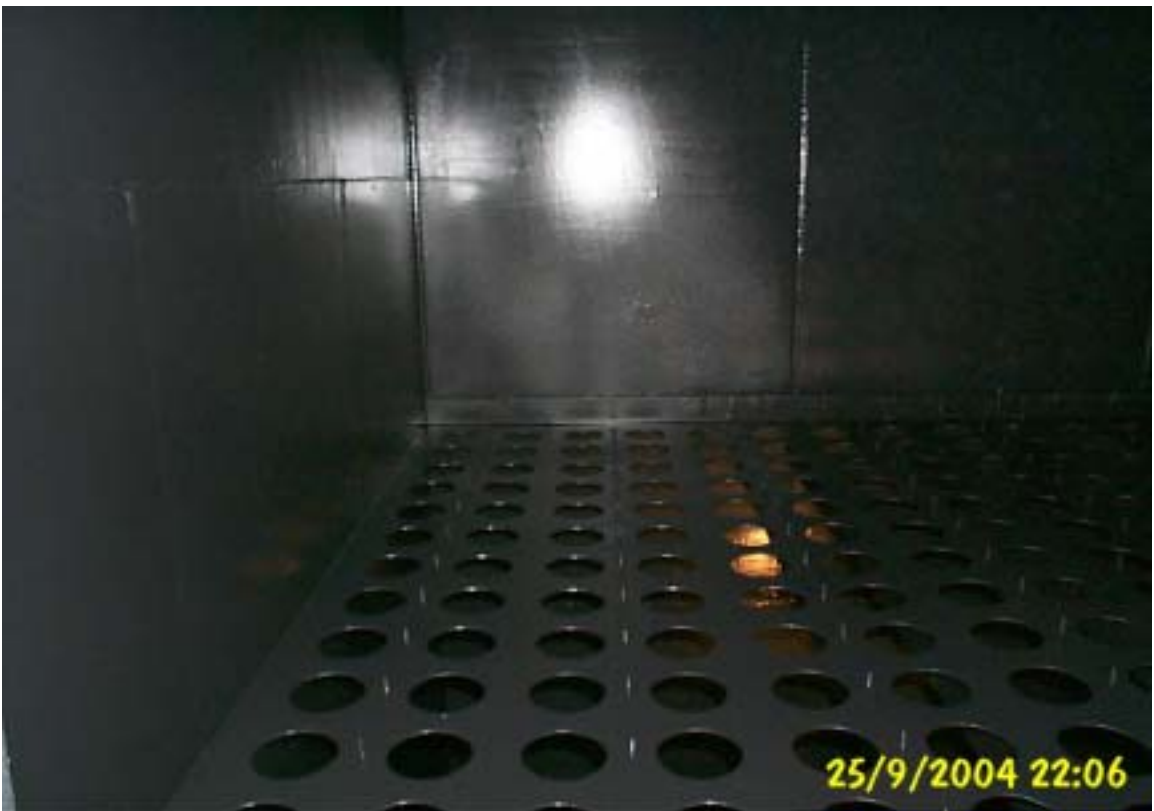
Figure 5. Baghouse protected from corrosion with FlueGard-225
