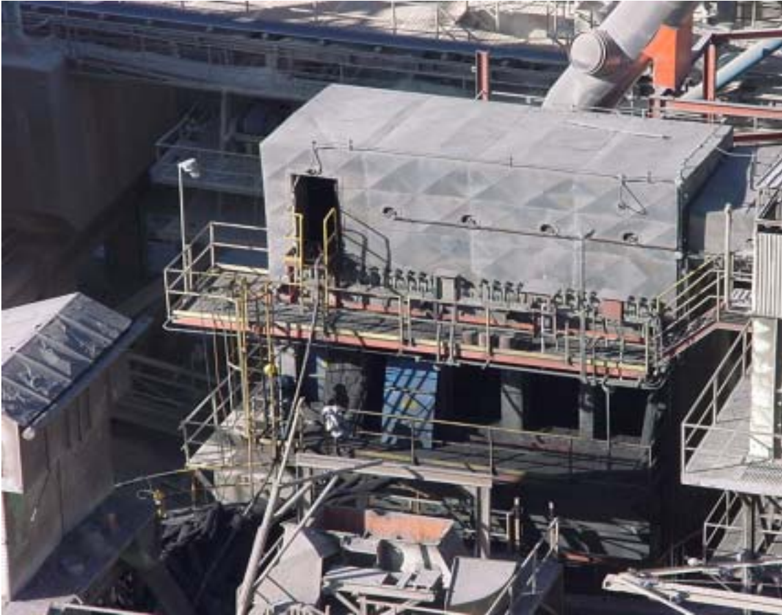
Figure 1. View of the Corroding Coke Mill Baghouse
