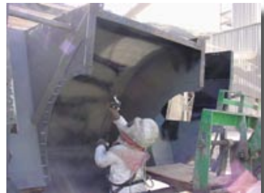
Figure 4: Coating of a fan housing to protect it from abrasion-corrosion.
