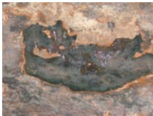
Figure 3: Kiln shell corrosion under the refractory, up to 8mm in thickness.
